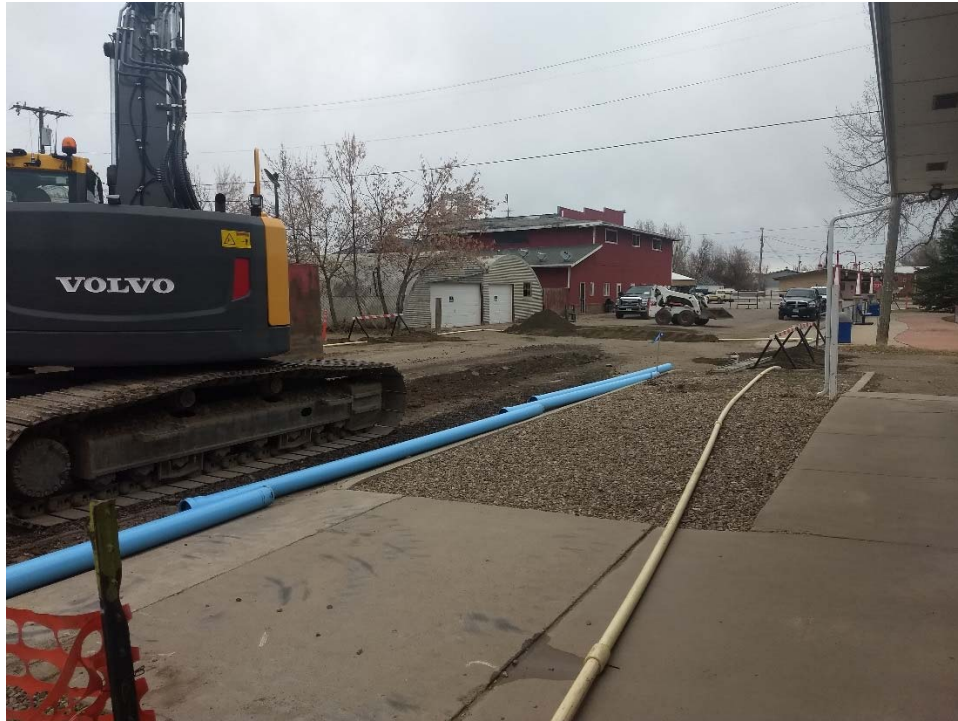
Temporary water piping along 1 st Street
